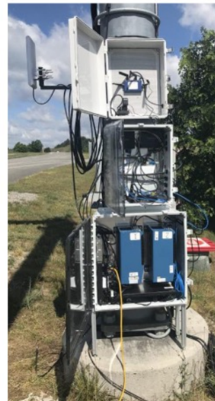
5G UE, PoE Hub, Mgmt Switch, Edge Servers
