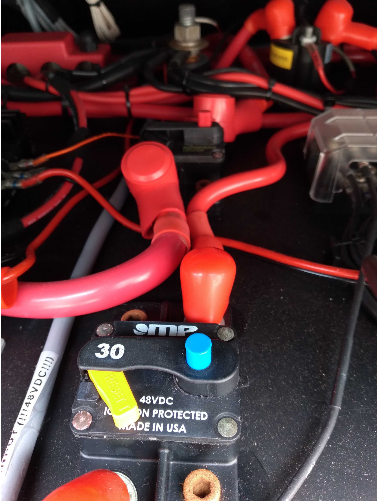
Image 4: 2 breakers underneath on bottom shelf in cabinet
